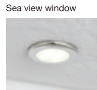
Room Light [Rest room]
